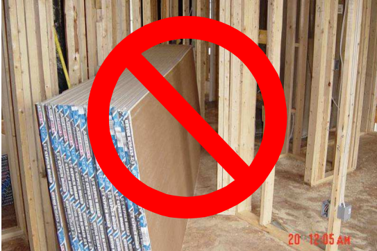
Gypsum stocked incorrectly on edge
