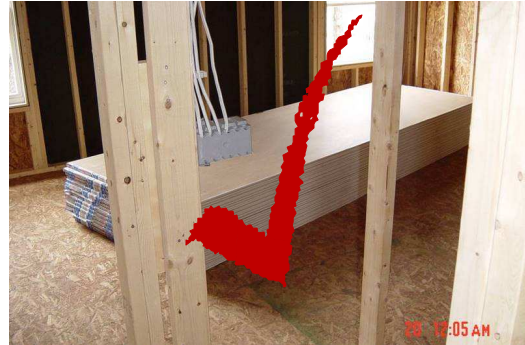
Gypsum stocked correctly flat and in center of room, maximum of 25 boards high
